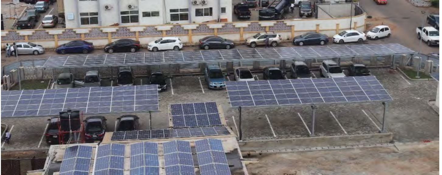
The 20 Bay Solar car park.
