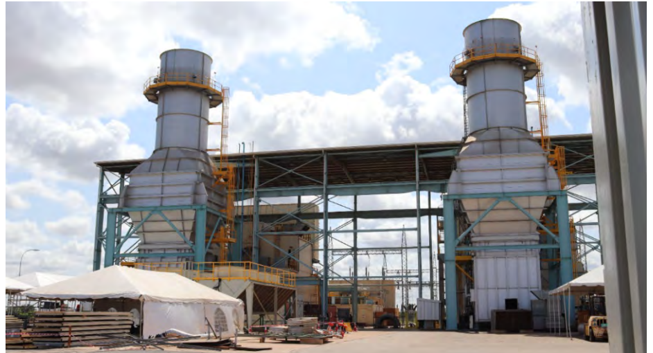
The Kpone Thermal Power Plant Gas Turbine Units
